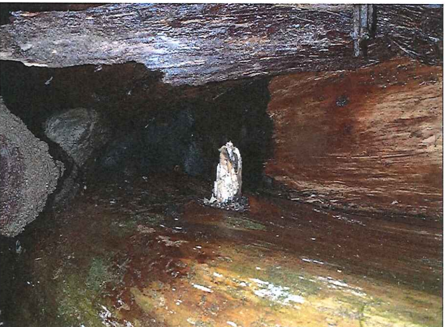
CK2264 wheel path fill failure
