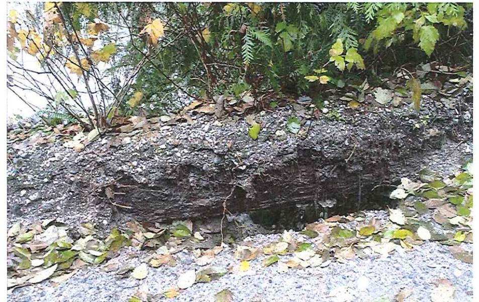
CK2264 Downstream side deck failure
